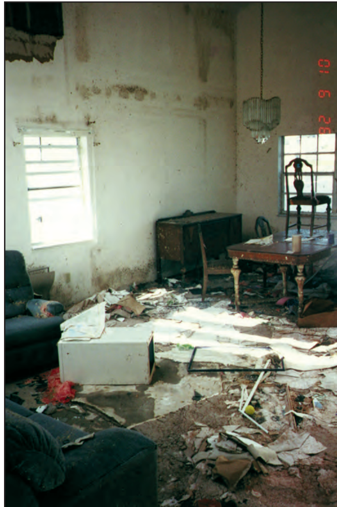
Figure 4 In low-lying areas, wind and rain damage to interior finishes and furnishings was exacerbated by flood waters.
